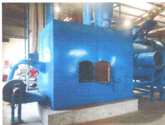
Hot air stove
