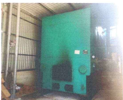
Thermal oil furnace
